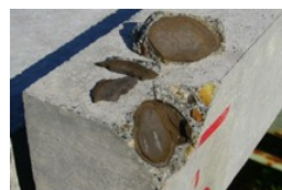
Figure 3: Outdoor exposure test of concrete containing aggregates that are weak for the freeze-thawing action
