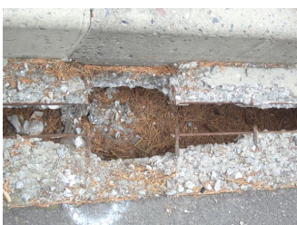
Photograph-2 Precast concrete product deteriorated by DEF
