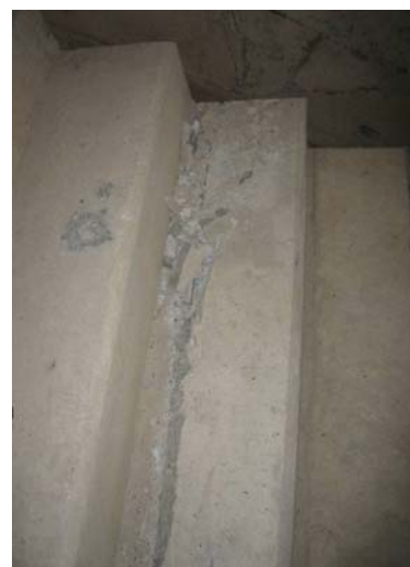
Photo. 4 Cracks in concrete steps along contraction joint J-8 in the gallery
