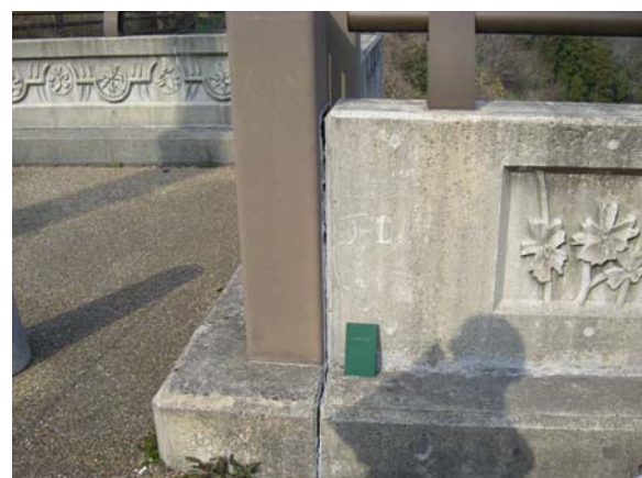
Photo. 2 Opening of crest parapet joints on contraction joint J-1
