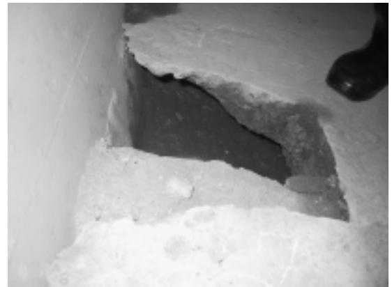
Figure 4. Detail of failure occurred at junction between tunnel invert and sidewall foot in Tunnel B.
