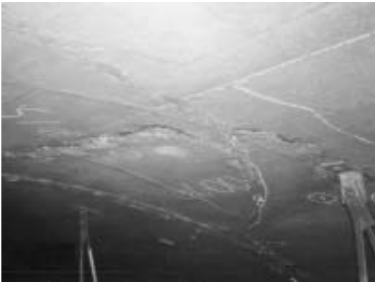
Figure 2. Detail of failure occurred at tunnel crown in Tunnel A.
