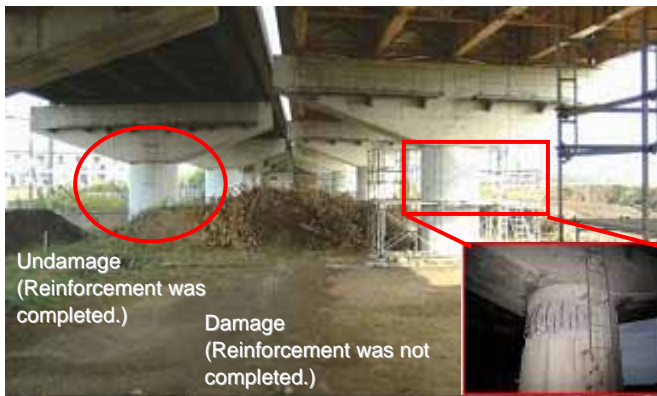
Figure 12 Undamaged and damaged piers next to each other during the 2004 Niigata Chuetsu earthquake (Mj6.8), in which undamaged piers were reinforced in the middle of the seismic reinforcement program by the administrator
