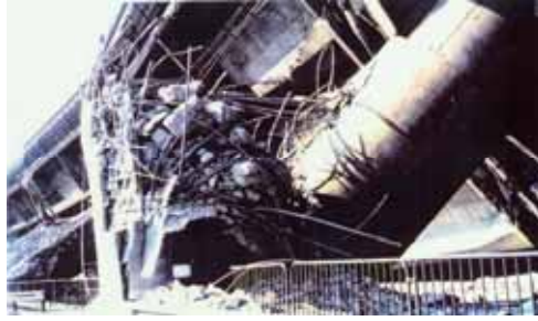
Figure 11 Collapse of a highway viaduct of Route 3, Kobe route, of Hanshin Expressway during the 1995 Hyogo-ken Nanbu earthquake
