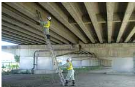
Figure 6 Typical bridge inspection. Visual inspection is the standard in the current routine inspection practice.
