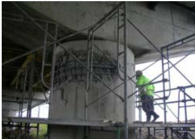
Photo 8 Damaged Pier P5 (Before Retrofit)
