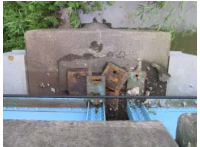
Photo 4 Damage of Bearings
