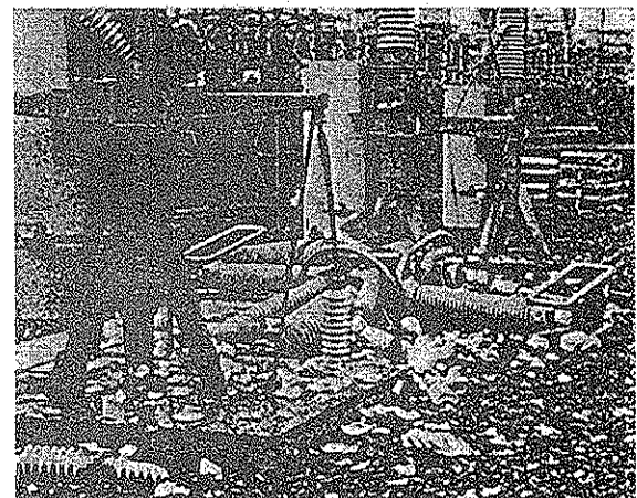
Photo. 2 Damage of Power Plant
