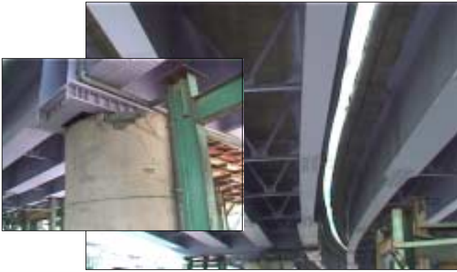
Figure 9. Shear racking on eccentric connections
