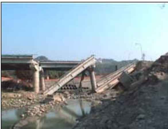
Figure 5. Spans collapsed of Shi-wei Bridge
