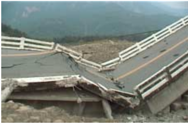
Figure 10 Spans collapsed of Tong-tou Bridge
