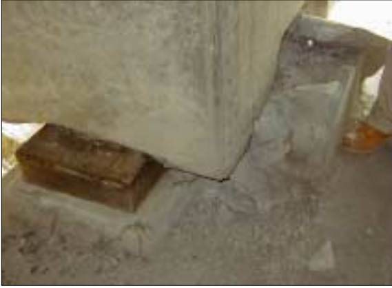
Figure 3. Shear keys failure in Sakarya Viaduct
