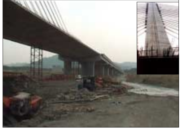
Figure 6. Cable fracture of a cable-stayed
