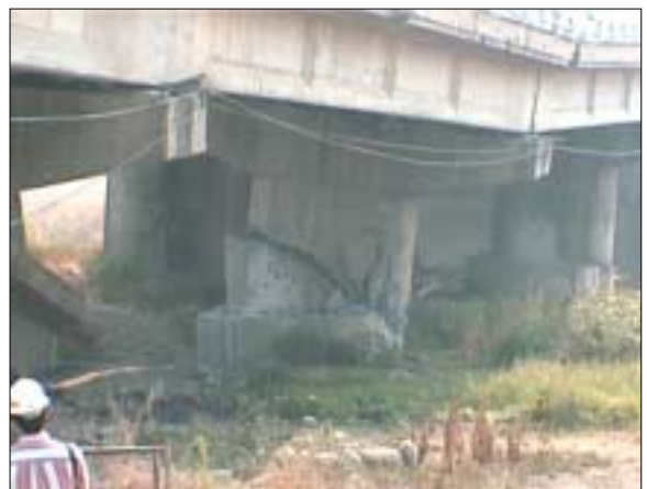
Figure 8. Pier shear failure of U-Shi Bridge
