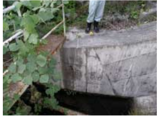
Photograph 11 Cracking on the Spillway Channel Wall of the Uh Dam
