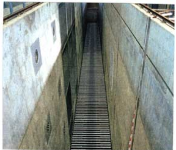
Figure 5. Array of water supply pipes at the bottom of the LHGF.
