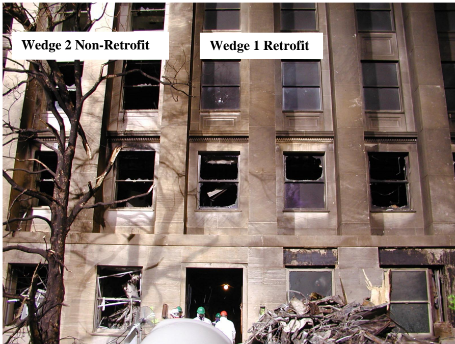
Figure 4. Exterior view of transition between Wedge 1 (on right, retrofit) and Wedge 2 (on left, non-retrofit). First floor non-retrofit window adjacent to transition may be High Hazard blast response. Second and 3 rd floor fire damage. Approximately 135 ft (44.2 m) North of plane impact point.
