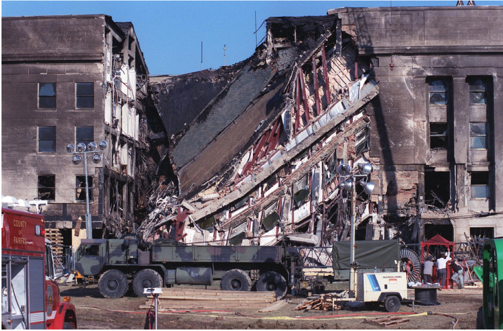
Figure 3. Collapsed section/plane impact area in Wedge 1. Plane entered the 1 st floor at an angle of approximately 40 degrees from perpendicular moving toward the left into Wedge 2.
