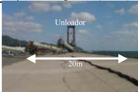
Fig-9 Damaged Quaywall in Sakai Port
