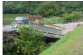
(a) Overview of Damage
