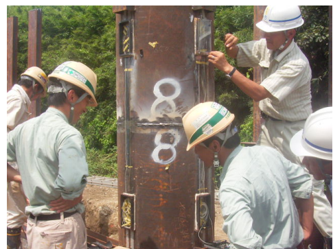
Fig.4 Welded connection between bottom and top pieces of pile and treating optical fiber
