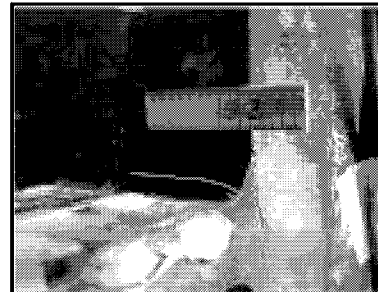
Photo 2 A fatigue crack on steel member
