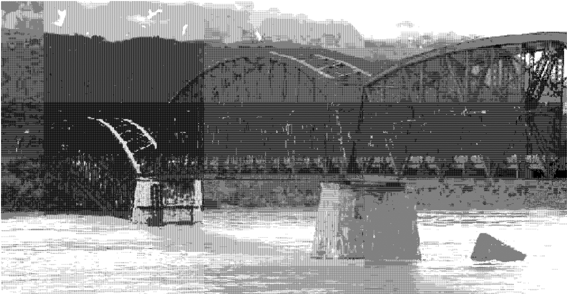
Figure 1: The Million Dollar Bridge, Showing Piers 2 & 3 and the Fallen Span 4.
