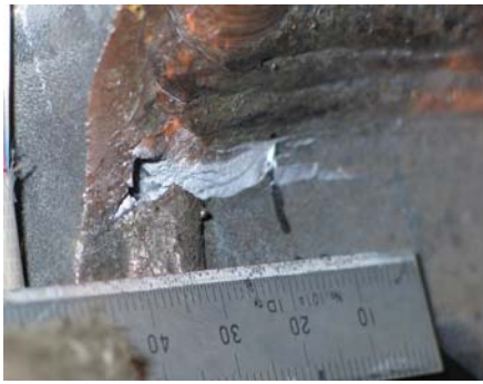
Fig.14 Cracks propagation into web plate in C2(-4 \delta_y )
