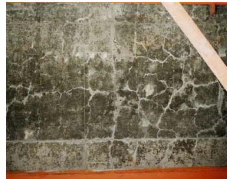
Fig. 3.12: CRACKS IN CONCRETE DECK
