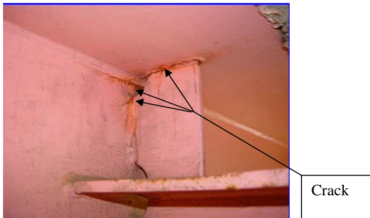
Fig. 3.9: OCCURRENCE OF A CRACK ON A COMPOSITE STEEL GIRDER BRIDGE
