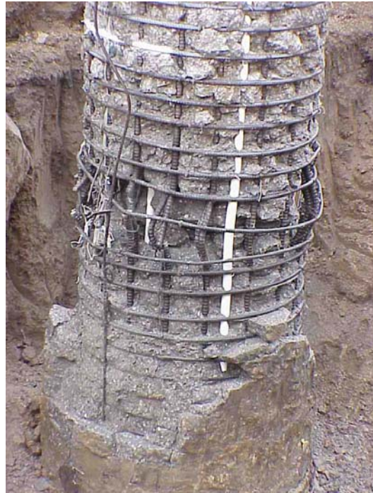
FIGURE 3 - HOOP FRACTURE AT MAXIMUM DUCTILITY.
