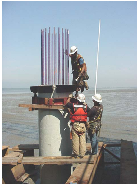
FIGURE 8 - COLLAR PLACED AT TOP OF COLUMN TO SUPPORT PRE-CAST BENT CAP BEAM.
