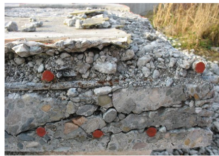
Photo 5 Cut section of the bridge deck slab (directly below the wheel travel position)
