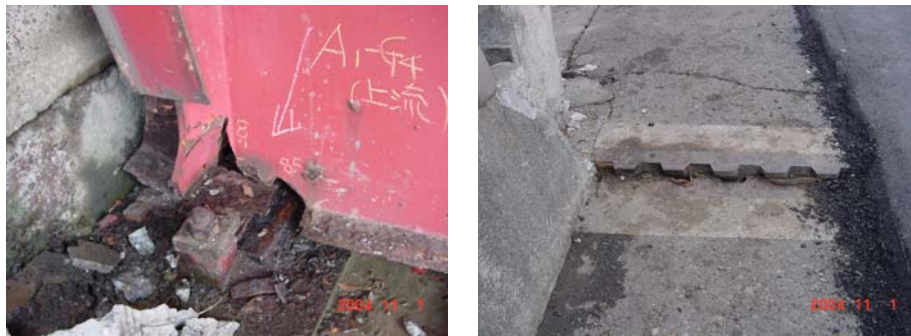
FIGURE 8. RUPTURE OF CORRODED PART OF THE GIRDER EDGE AND BUMP CREATED BY THE FALLEN GIRDER (NIIGATA-CHUETSU EARTHQUAKE)
