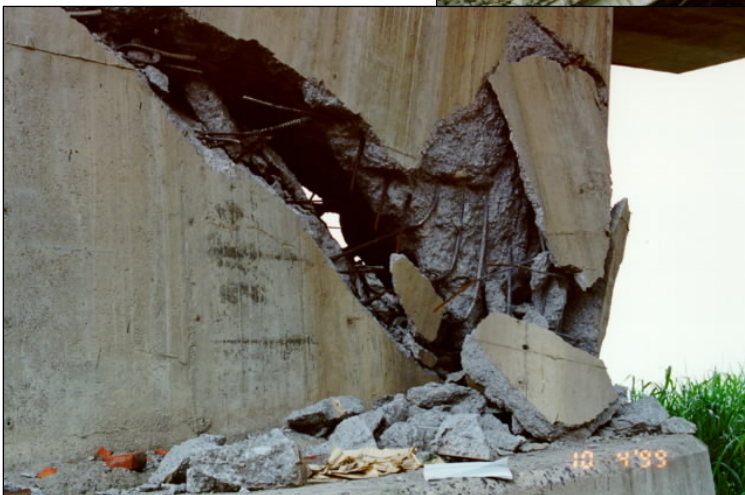
Figure 4 (left). Diagonal shear crack in lightly reinforced concrete pier of the Wu Shu bridge in Taichung.
