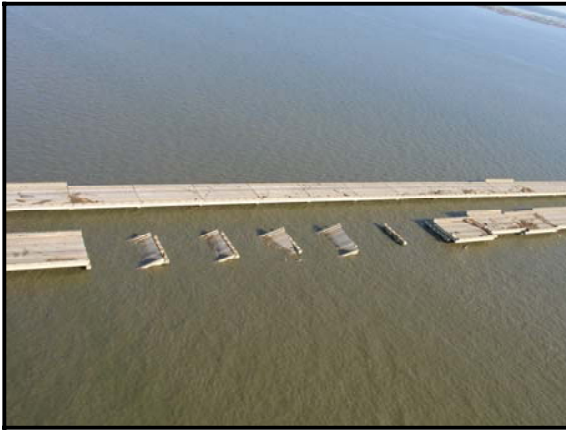
Figure 20 – Damage due to diagonal wave action
