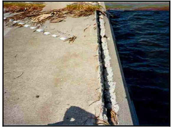
Figure 23 – Damage to bridge railing
