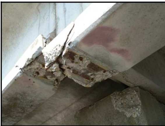
Figure 22 – Damage to girder ends
