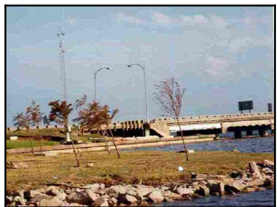
Figure 6 – Bridge Abutment Scour
