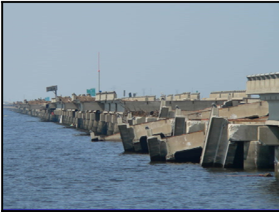
Figure 21 – Damage due to wave action
