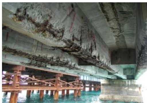
Fig. 1 Corrosion of reinforcements
