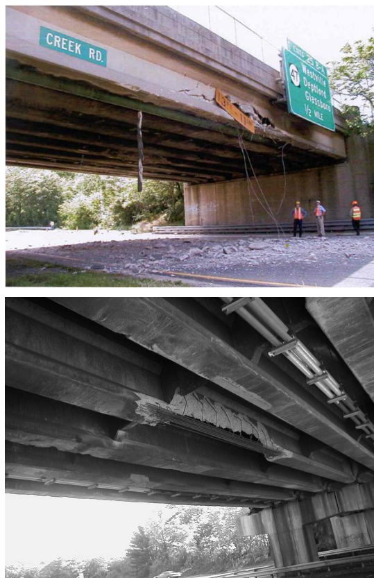
Figure 1 Exposed Prestressing Strands of Damaged Interior and Fascia Girder of Creek Road Overpass Bridge
