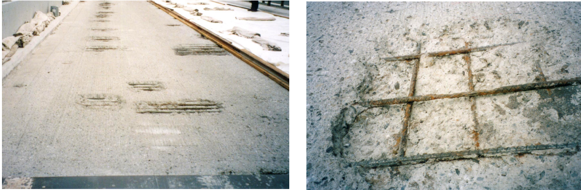
Fig. 4 Corrosion of top mat reinforcement due to salt use in reinforced concrete decks Both photo shows top of decks after asphalt and spalled concrete cover were removed.
