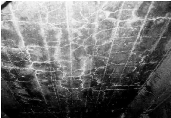
(a) Grid cracks
