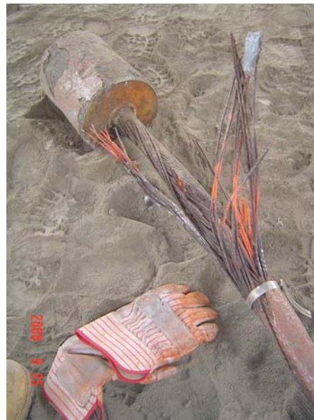
Figure 3 – Photo of Deteriorated Suspender Strand with Broken Wires (After Removal)
