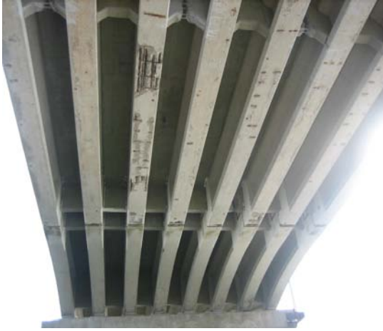
Figure 4 – Damaged prestressed girders
