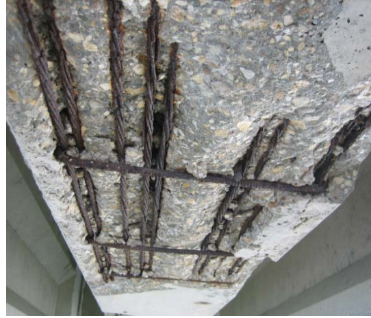
Figure 5 – Close-up of recovered girder
