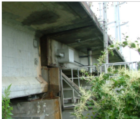
(a) Salt Damage
