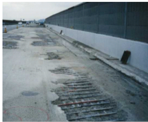
(b) Salt Damage (RC Deck)
