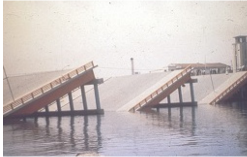
Photo1 Damage of pile bent pier bridge the 1964 Niigata Earthquake
