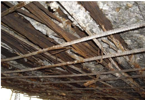
Photo 5 Corroded and Broken PC Cables in Precast Segment Box Girder Bridge
