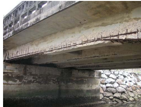
Photo 2 Concrete Bridge with Cover Concrete Fell Off
