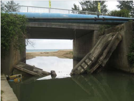
Photo 1 Collapsed Concrete Bridge in Okinawa
