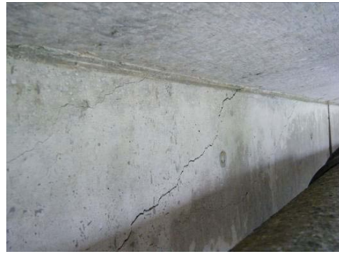
Photo 4 Diagonal Crack at the End of PC Hollow Bridge Girder
