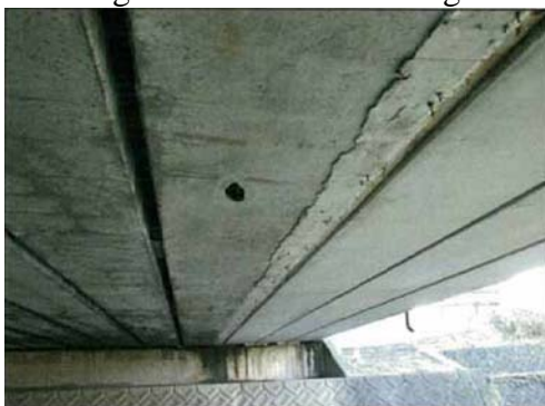
Photo 7 Void in Bottom Flange of Precast Hollow Girder
