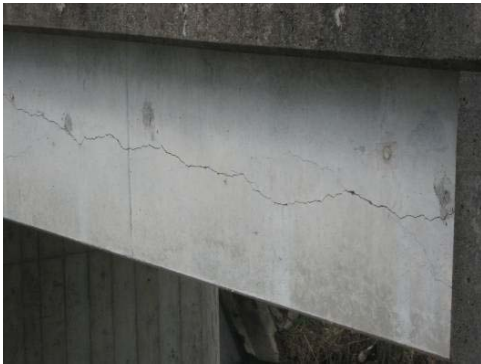
Photo 3 Horizontal Crack on Precast Hollow Girder
