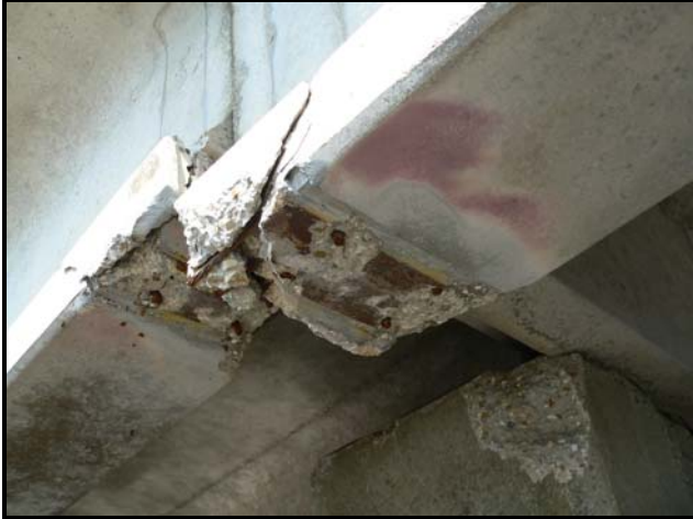
Figure 22 – Damage to girder ends
