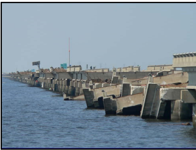
Figure 21 – Damage due to wave action
