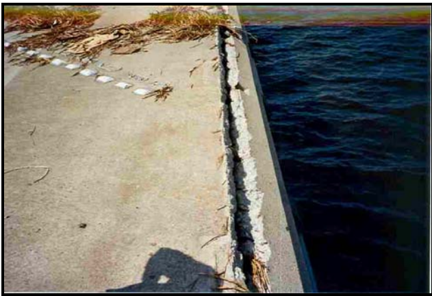
Figure 23 – Damage to bridge railing
