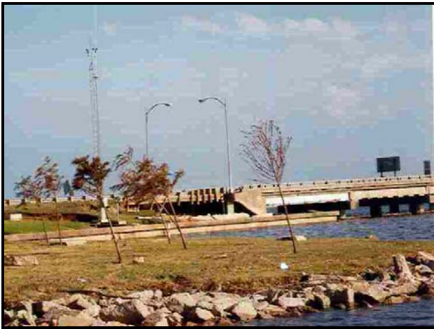
Figure 6 – Causeway Bridge Abutment Scour
