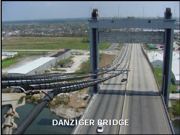
Figure 14 – Droop Cables on Vertical Lift Bridges
