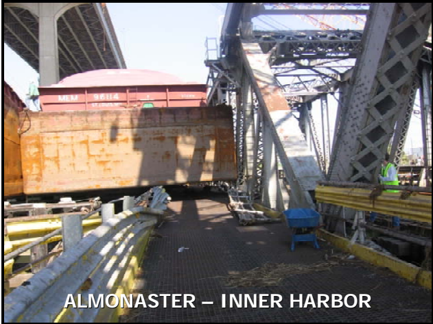
Figure 16 – Debris on Structures
