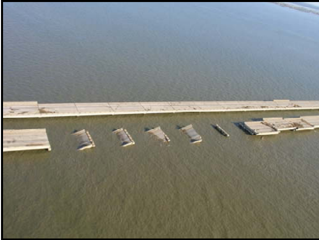
Figure 20 – Damage due to diagonal wave action
