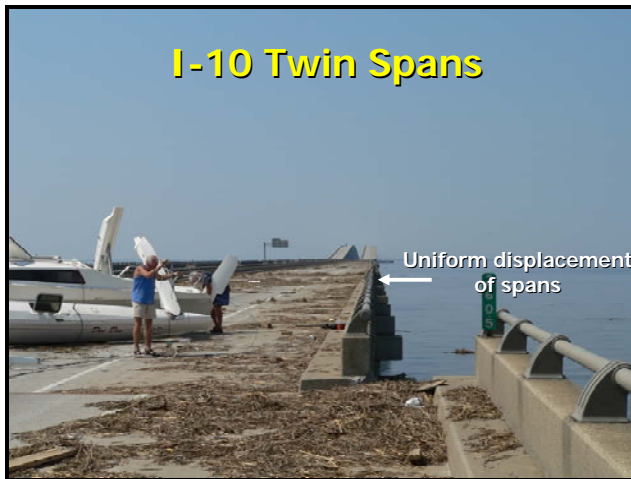
Figure 19 – Damage due to transverse wave action
