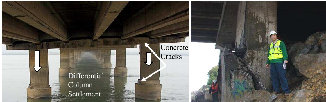
(a) Uneven settlement and induced damage (b) Shear failure in upstream column FIG. 15 DAMAGE DUE TO UNEVEN SETTLEMENT AND SLOPE FAILURE
