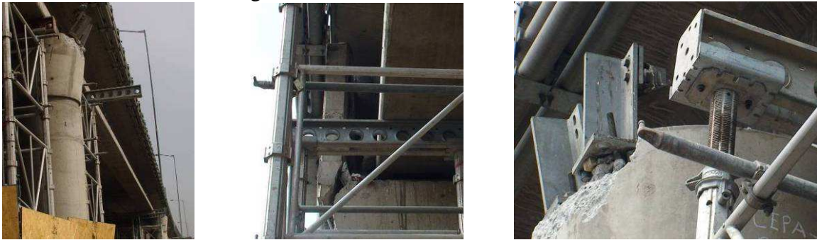
(a) Overall damage (b) Curtain wall at the west abutment (c) Damage to steel stoppers FIG. 6 DAMAGE TO THE EASTBOUND INDEPENDENCIA BRIDGE
