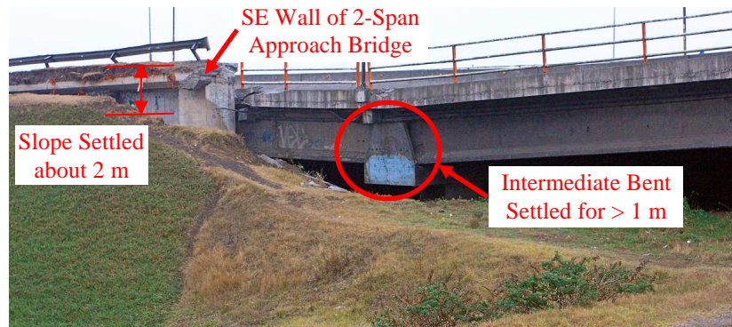
(c) Intermediate bent settlement of approach spans
