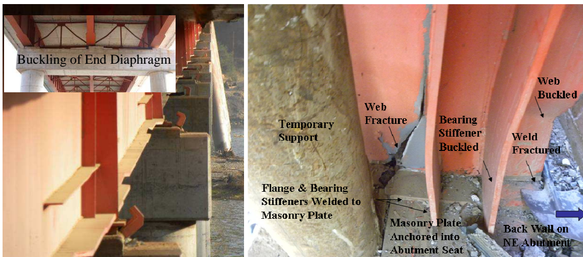
(a) Girder offset and cross frame buckling (b) Girder damage at north abutment
