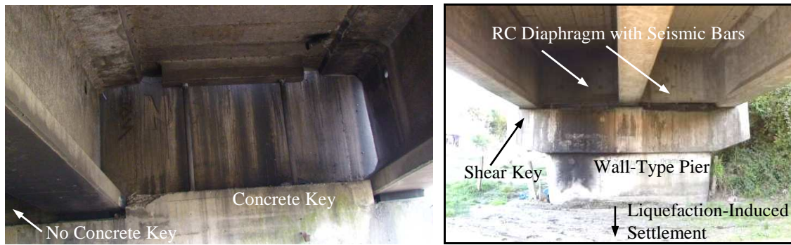
(c) Llacolén bridge with concrete key (d) East Ramadillas bridge with full diaphragm
