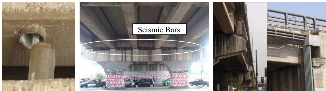
(a) Displaced seismic bar (b) Typical flared wall pier (c) Damage of shear keys FIG. 7 DAMAGE TO THE WESTBOUND INDEPENDENCIA BRIDGE
