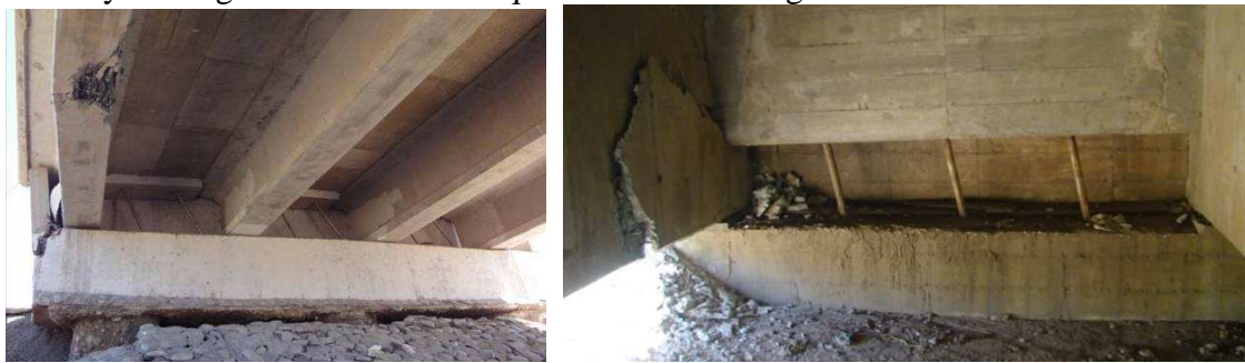
(a) Chada bridge with no diaphragms (b) San Nicolás bridge with partial diaphragms
