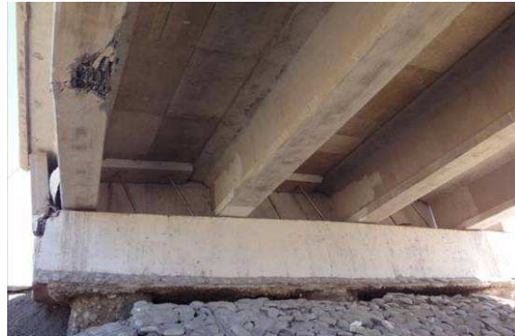
(b) Bottom flange damage
