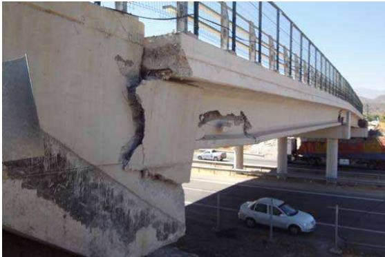
(a) Curtain wall shear failure at abutment
