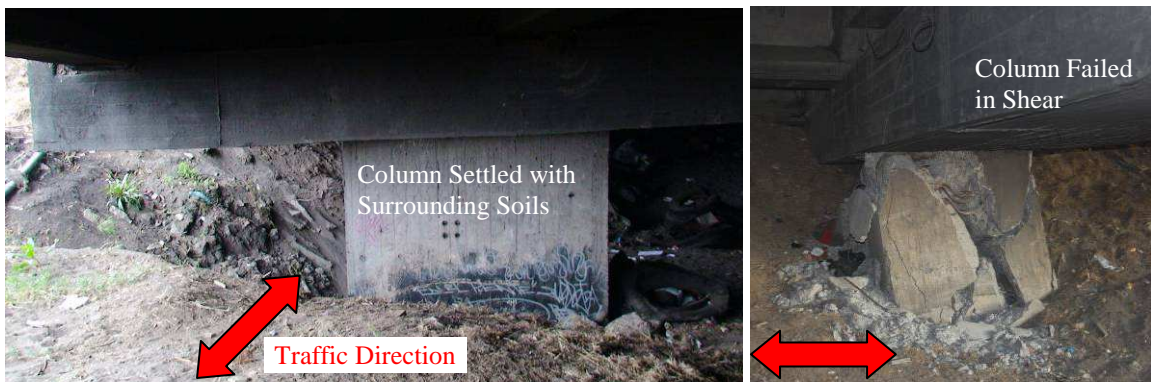
(a) Column settlement (cracks on far side) (b) Reduced column height due to shear failure FIG. 14 DAMAGE TO INTERMEDIATE BENT OF APPROACH SPANS
