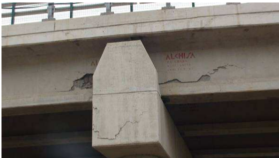
(c) Curtain wall damage at bent
