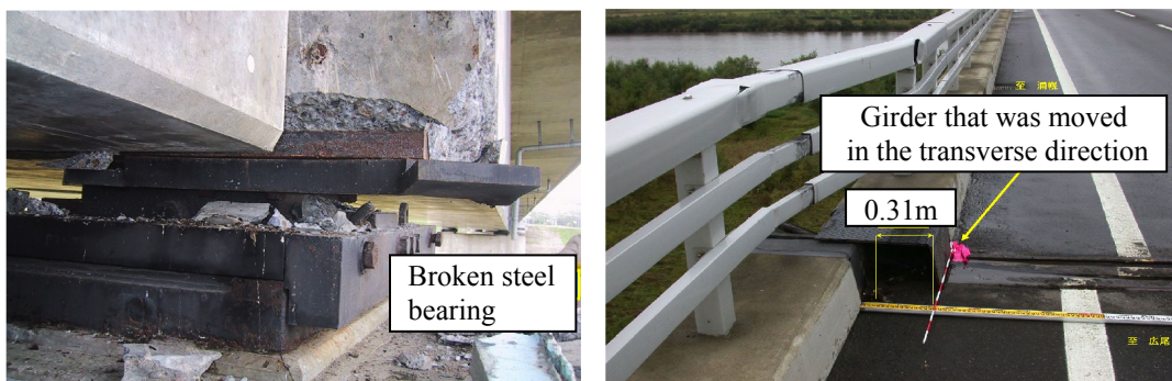
Photo.2 Damage situation of Tokachi-kakou Bridge
