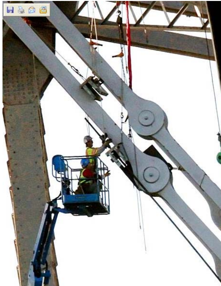
FIGURE 3-THE ORIGINAL FIX INVOLVED THE USE OF HIGH-STRENGTH RODS TO BYPASS THE CRACK.
