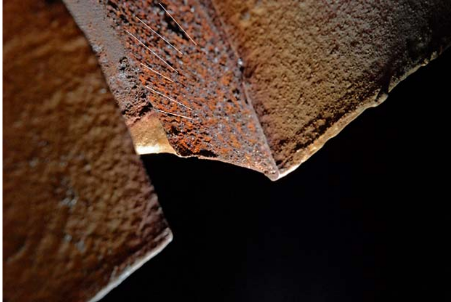
FIGURE 7-CLOSE-UP OF FRACTURE SHOWING RADIAL RIDGES POINTING TO LOCATION OF CRACK INITIATION.
