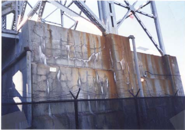
Figure 3. A view of the north side of the abutment at the start of the project
