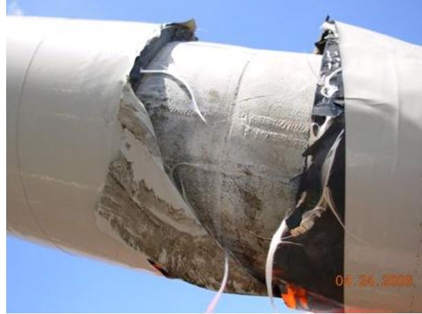
FIGURE 7- PE JOINT SEPARATION
