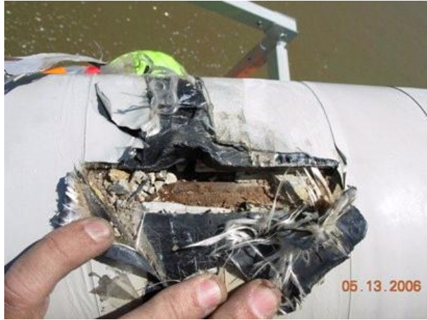
FIGURE 6- CORROSION OF WIRES AT PE SPLIT
