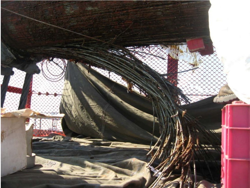
Figure 1: Broken wires in a suspension bridge main cable
