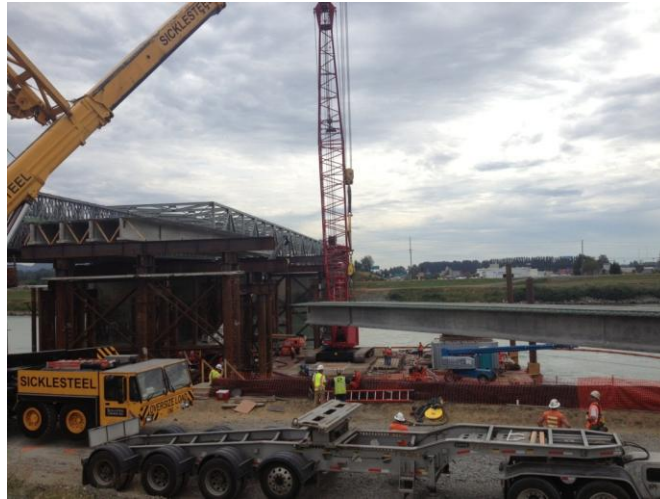
Figure 5: Permanent superstructure constructed on a steel piling and bents downstream of the temporary spans
