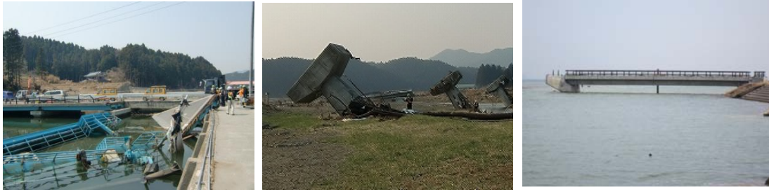
Photo 1. Examples of damaged bridges due to the 2011 Tohoku Earthquake Tsunami (From Left to Right: Washout of superstructure, Collapse of piers, and Washout of backfill behind abutment)
