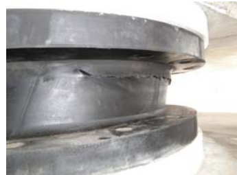
(b) Crack of rubber bearing
