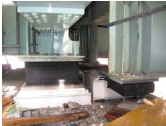
(a) Rupture of rubber bearing
