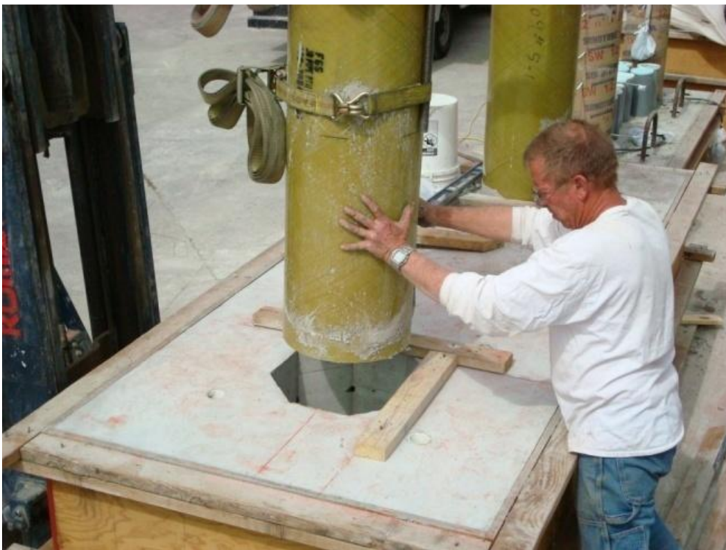
Fig. 10 – Precast concrete filled FRP tube column placed in precast footing at the University of Nevada - Reno
