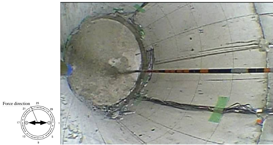
(b) Damage observed at inside face
