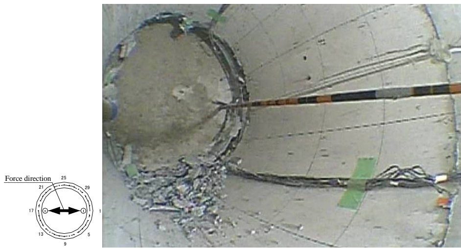
(b) Damage observed at inside face
