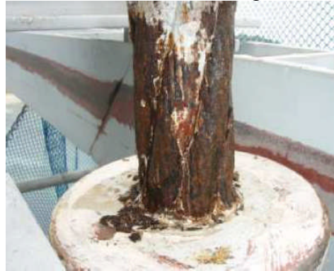
Photo 4 Corrosion of Suspender Rope Near Anchorage (Ohnaruto Bridge)
