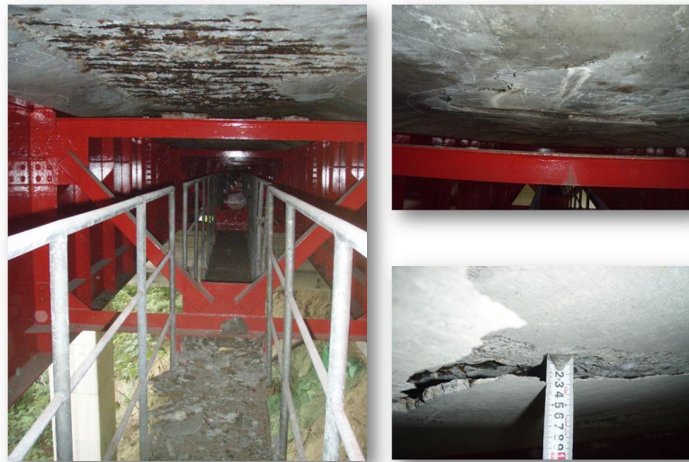
Pic. 1 Deck deterioration situation
