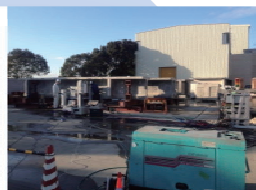
Generator and Linac and bridge
