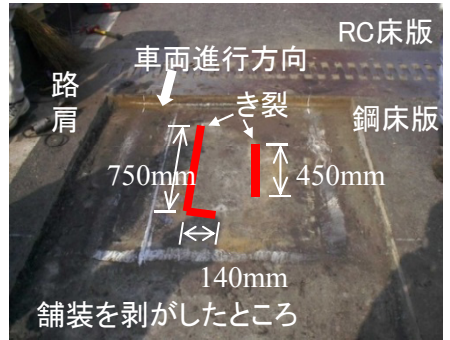
鋼床版表面のき裂
