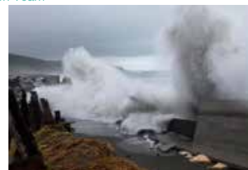
Damage to coastal revetments due to high waves
