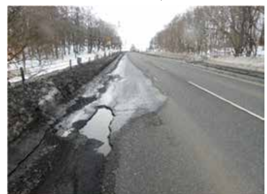
Pavement distress caused by freeze-thaw cycles
