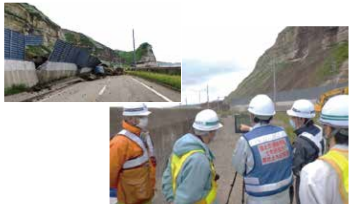
June 2021 rock slope failure on National Route 229: On-site meeting with road administrators (photographed on June 7, 2021)
