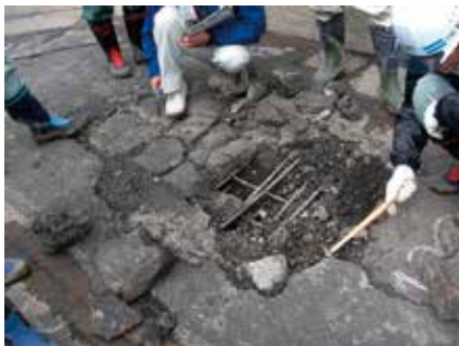
Gravel formation and collapse of road bridge RC slabs due to frost damage
