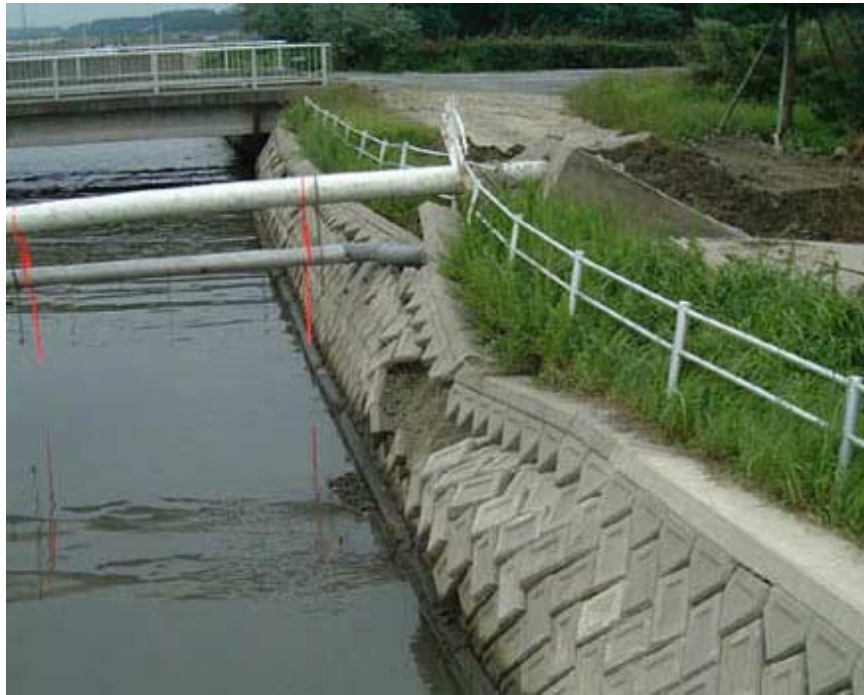
Photo 5 Distorted revetment and Yumeminato bridge
