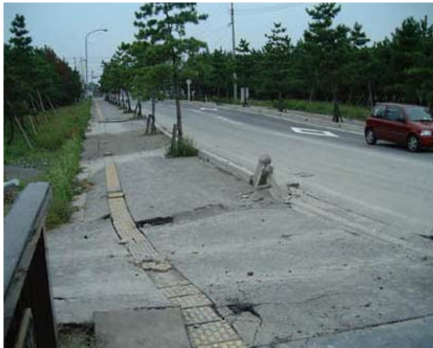
Photo 4 Distortion of road shoulder concrete blocks due to ground displacement, near the Yumeminato bridge
