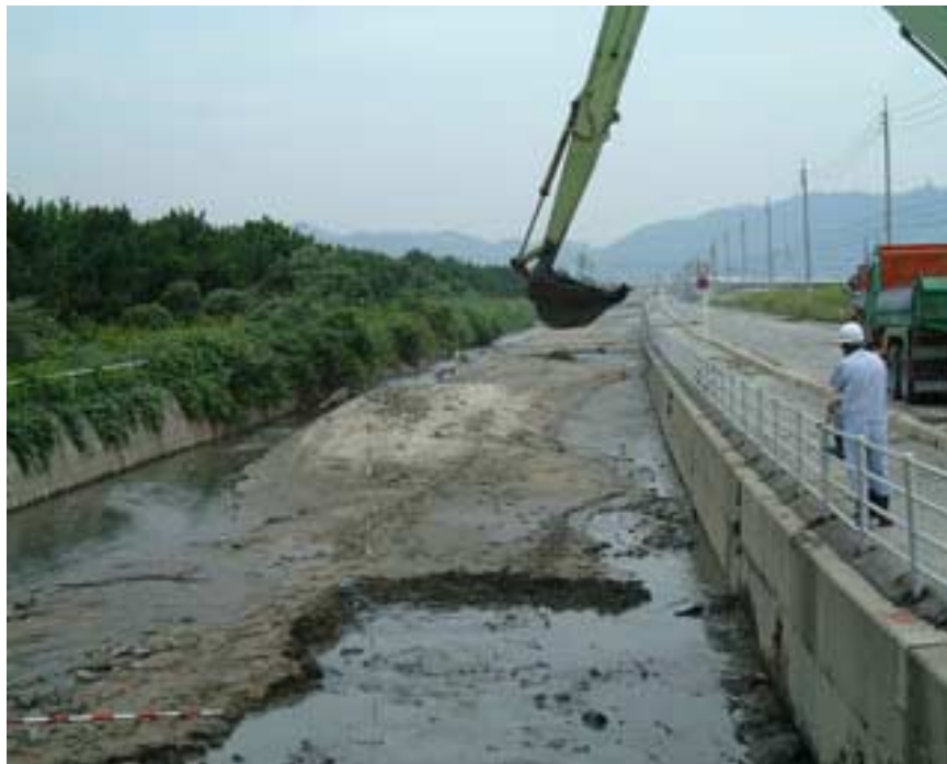
Photo 5-2 Extensive amount of sand boiling at Takematsu-gawa (Looking from Yumeminato bridge)
