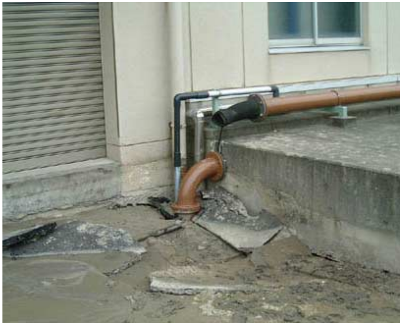
Photo 7 Settlement of the ground and associated breakage of pipes, Sakai-minato Sewage Treatment Center
