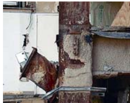
Photo 5. Fire protection at Bunker Trust Building
