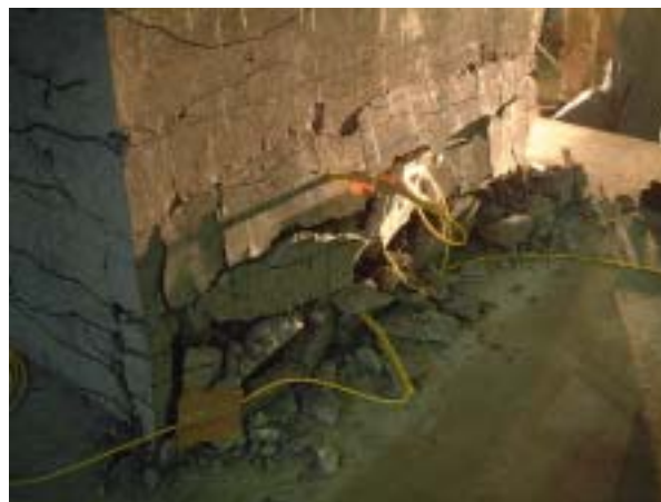
(b) Damage at the Bottom of Column
